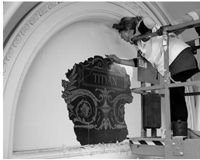
Paint being removed from the lunettes in Room 32 to reveal the original Victorian decoration beneath
